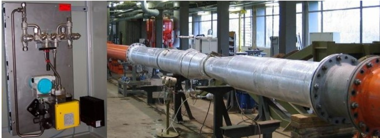
Steam billing measurement using a Venturi tube in accordance with DIN EN ISO 5167 METRA Energie-Messtechnik Speyer, Germany Medium: steam, mass flow 65 t/h, steam pressure 21 bar(abs), steam temperature 280°C
